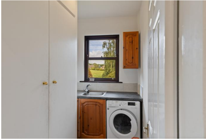
Utility Room 7'5" x 5'10" With plumbing for washing machine, stainless steel sink unit, cupboard housing the hot water tank and central heating boiler.
