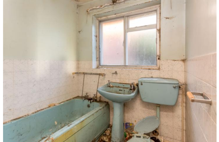
Bathroom 6'7" x 5'5" With 3 piece suite – note that the floor has collapsed in this room.
