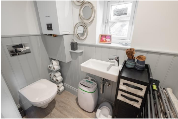
WC 5' 11" x 3' Comprising of a two-piece suite in white including a concealed flush WC and hand wash basin. The WC has an extractor fan, double-glazed window allowing a side aspect and it is home to the property's gas fired central heating boiler. The ground floor WC has similar panelling to half height.
